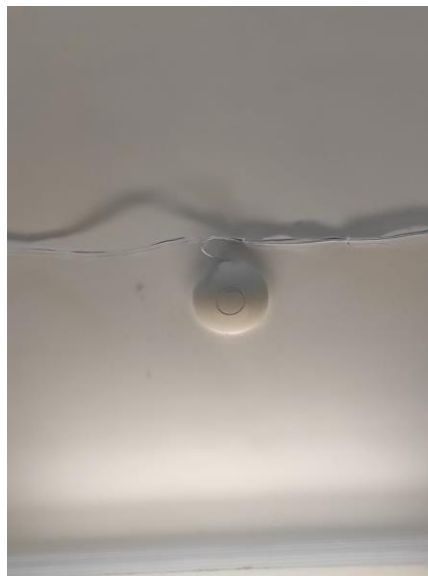
Gambar 3.20 Lab Industri Access Point 1
