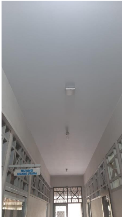
Gambar 3.8 Dekanat Access Point 2
