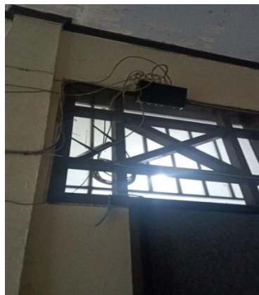
Gambar 3.24 Lab Mesin Access Point 1
