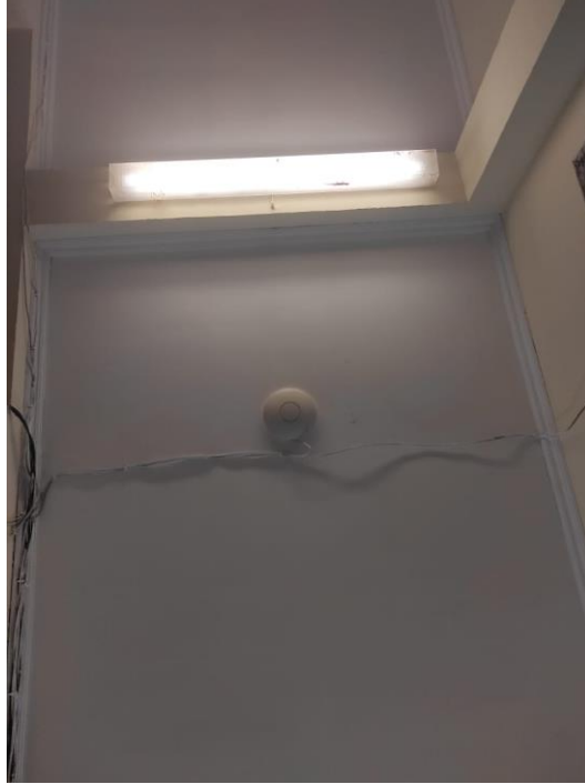
Gambar 3.21 Lab Industri Access Point 2
