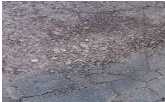
Gambar 2. 41 Pelepasan Butir ( Weathering/Raveling )
