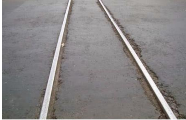
Gambar 2. 31 Rusak Perpotongan Rel ( Railroad Crossing )
