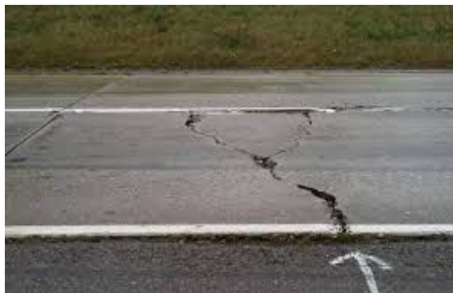
Gambar 2. 37 Patah Slip ( Slippage Cracking )
