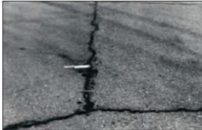
Gambar 2. 19 Retak Sambung ( Joint Reflec Cracking )
