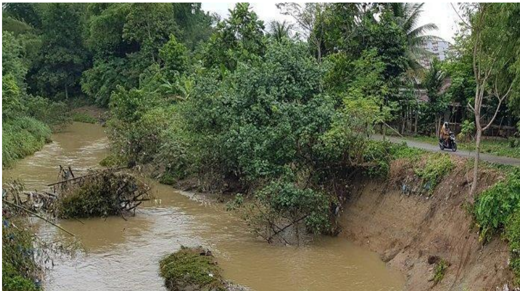
Gambar 2.9 Erosi Tebing Sungai
